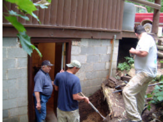
Bill Crawford, Syl Reitmeyer, and Steve McNelly work on the Retaining Wall at the Gatehouse.
