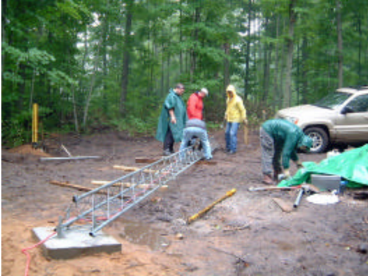
Setting up the new radio antenna tower was a muddy mess on the top of Hibb's Knob.
