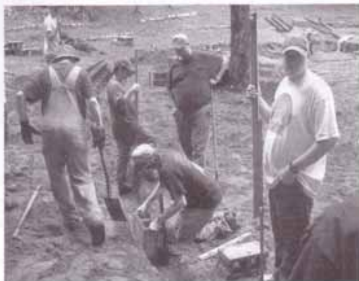
After marking out the proper size for the bowl and leveling the floor, a trench was dug and cinder blocks put in place.
