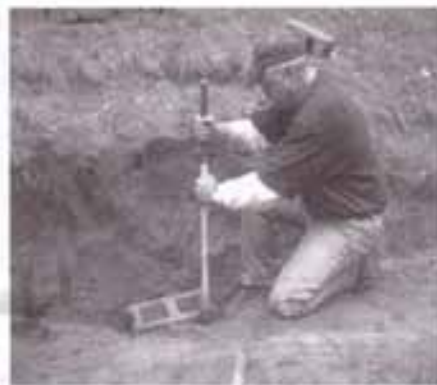
The first stone is placed on the first row. Cinder blocks will be use as a foundation
